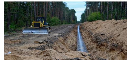
Domestic Transmission Pipeline
